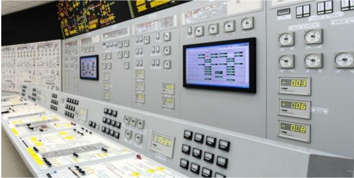
Reactor control panel, IAEA
